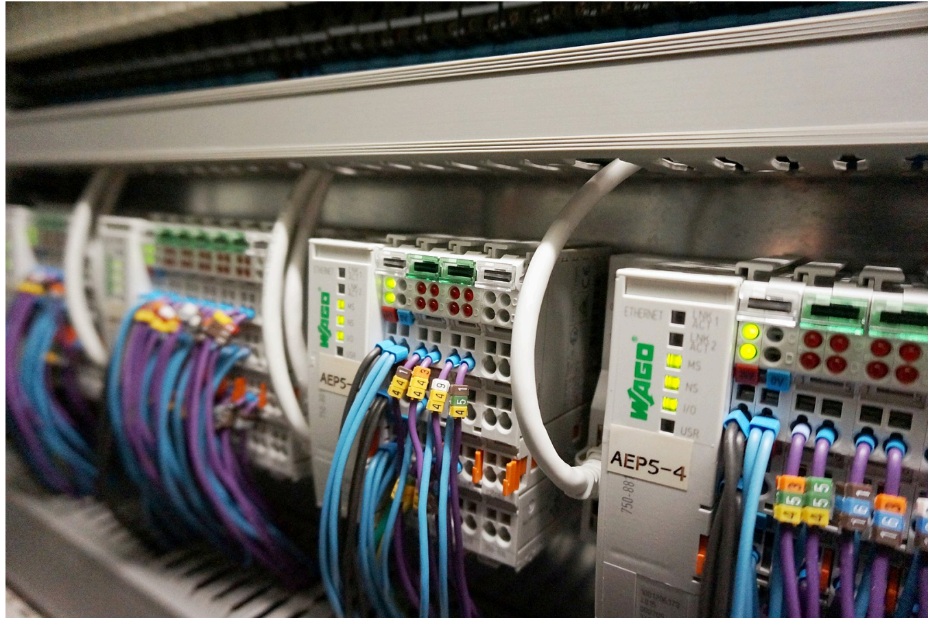
Figure 2: Programmable Logical Controllers A By Pierre75000 - Own work, CC BY-SA 4.0
